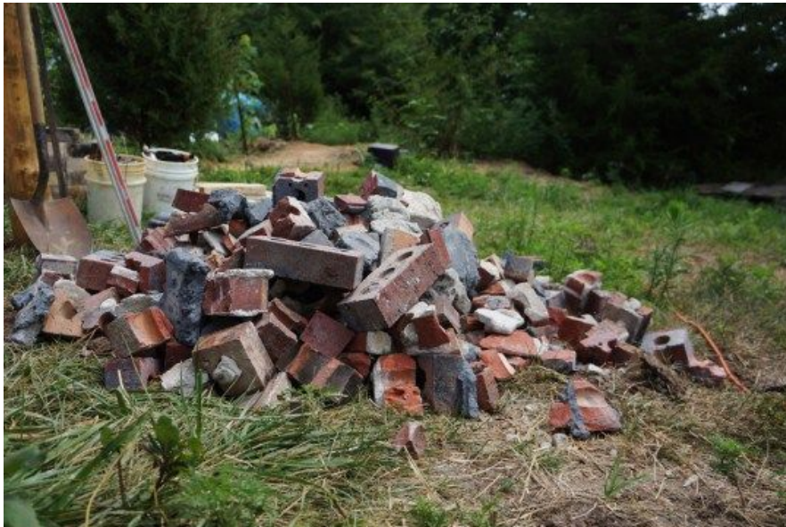
Junky rubble (broken bricks and cinder blocks, etc.) make for great fill in the center of the foundation
