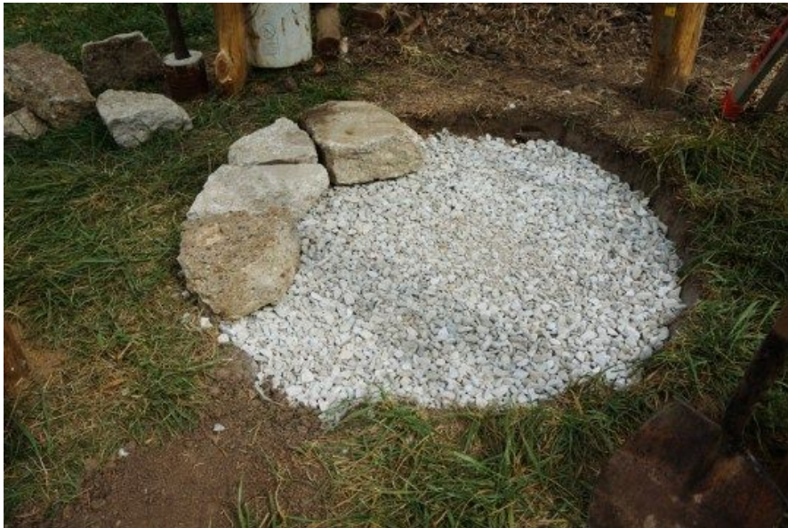
An 18" deep gravel bed for draining water away from the oven site — daylight drain is pictured in lower left corner and covered with soil
