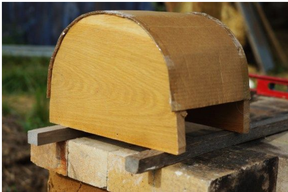
A simple doorway form. This will support the cob arch — note the 1" shim sticks
