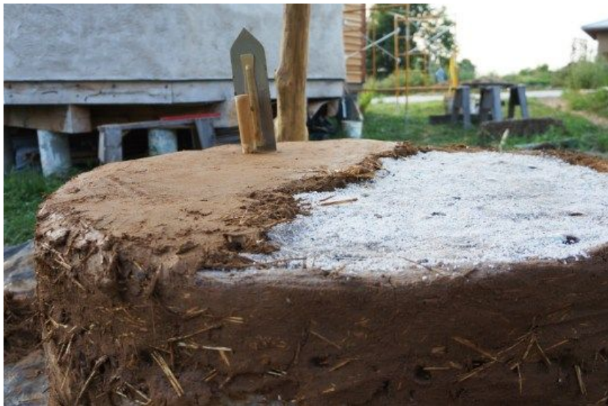
Using cob to make a thin, flat surface for the firebrick hearth — a trowel aids in smoothing the cob
