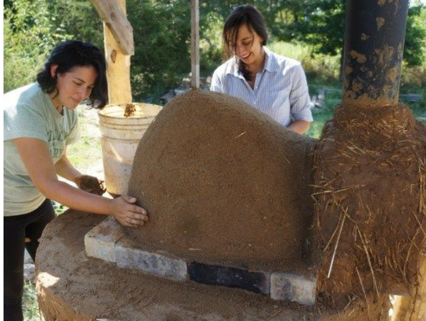
The nearly finished sand form, somewhat like an egg cut in half – note the stick with the 16" height mark
