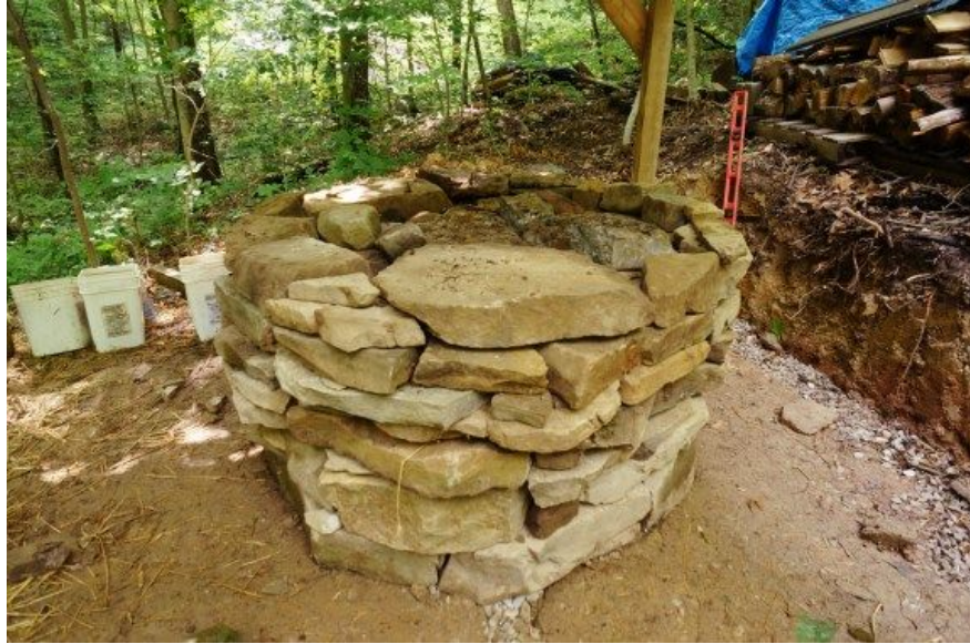
A 36" tall dry stacked stone foundation — this foundation represents quite a bit of material
